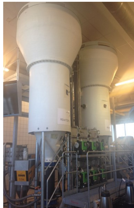
Figure 1 - Struvite reactors, Aaby WWTP
